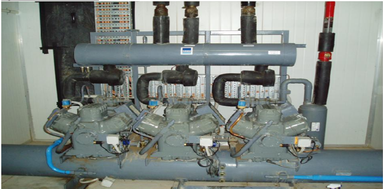
Figure 2 R22 Parallel Rack
