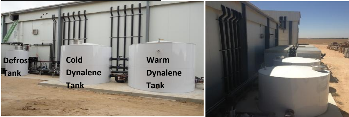
Figure.8 Secondary Refrigerant Tanks & Pumps
