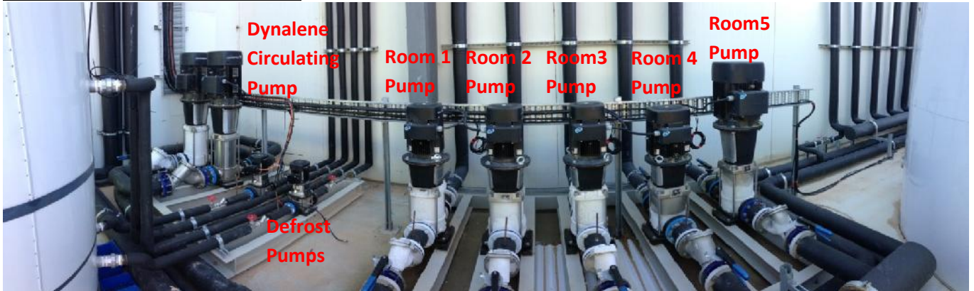
Figure.10 Dynalene Circulating Pumps
